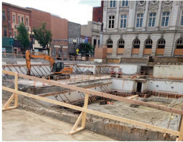
The courtyard area was fenced off in May so the initial demolition phase of the project could begin. The project started with the installation of shoring in the underground garage to brace the structure. Windows were covered in the surrounding structures to protect the glass. The base of the Civil War monument was also covered and the Greensburg Rotary town clock and art installations were temporarily removed for the duration of the project.
