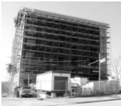
▲ This seven-story building located between North Main Street and North Pennsylvania Avenue will house employees from the Pennsylvania Department of Labor and Industry when completed next summer.
