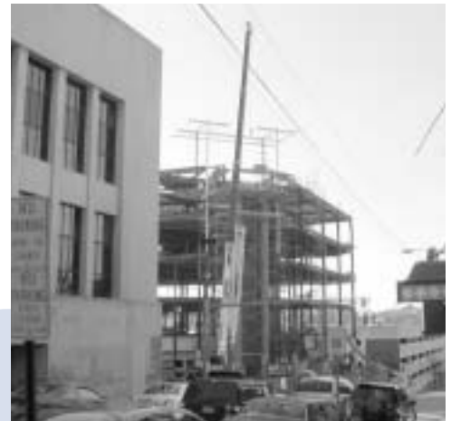
▲ Four floors are being added on to the existing Courthouse Square Extension on Pennsylvania Avenue in Greensburg.
